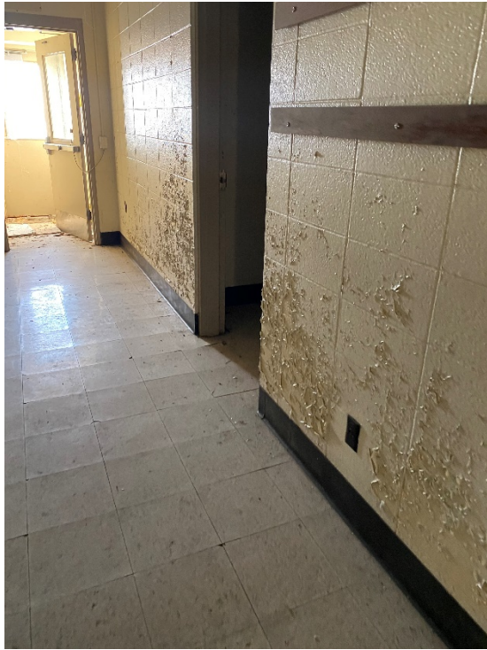
Photo 19 - View of peeling paint in Building 234
