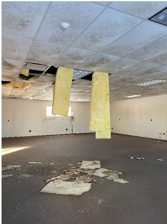
Photo 5 - View of ceiling tiles in Building 294
