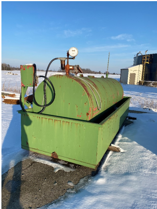
Photo 21 - View of fuel oil AST
