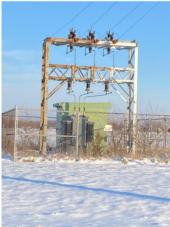
Photo 25 - View of pad-mounted transformer on South Farm
