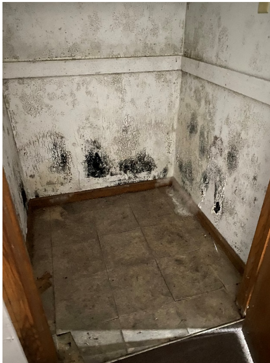
Photo 7 - View of mold and tile in Building 294
