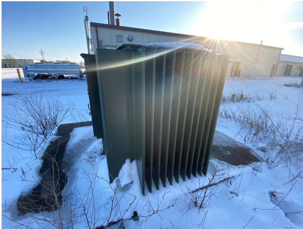
Photo 11 - View of pad-mounted transformer
