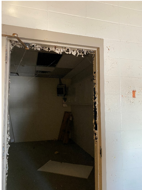
Photo 18 - View of peeling paint in Building 234
