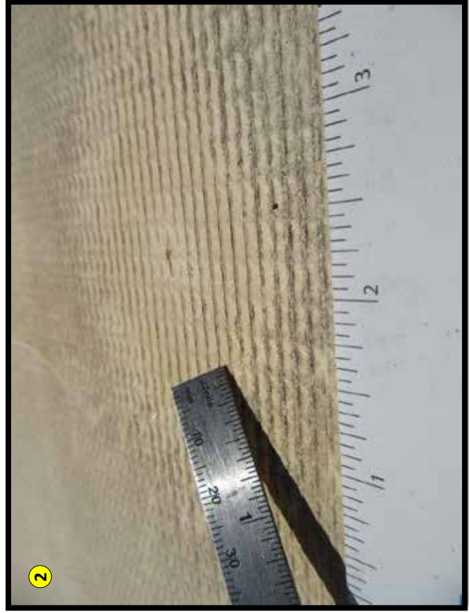
- Close View of Deteriorated EP Membrane
