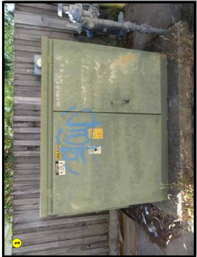
- View of Electrical Transformer in South Alley
