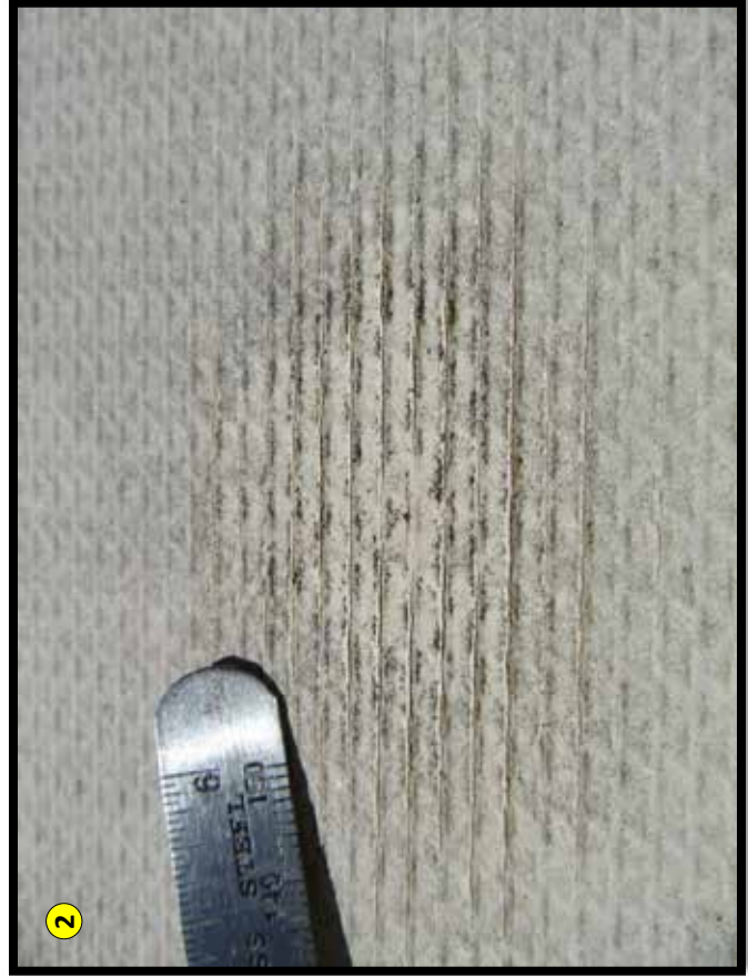
- View of Deteriorated EP Membrane
