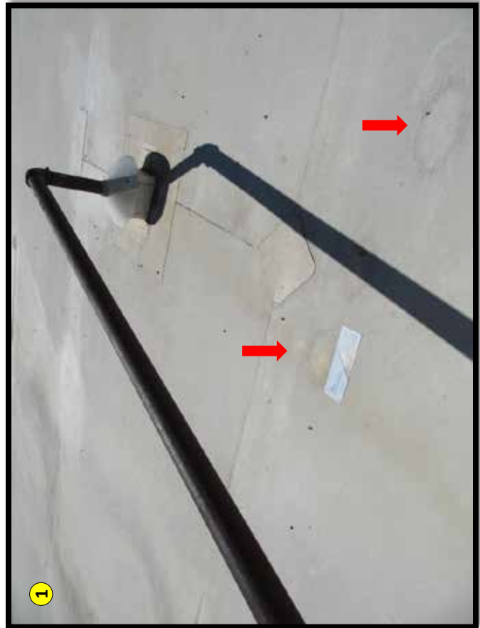
- View of Degradation to EP Roof Membrane
