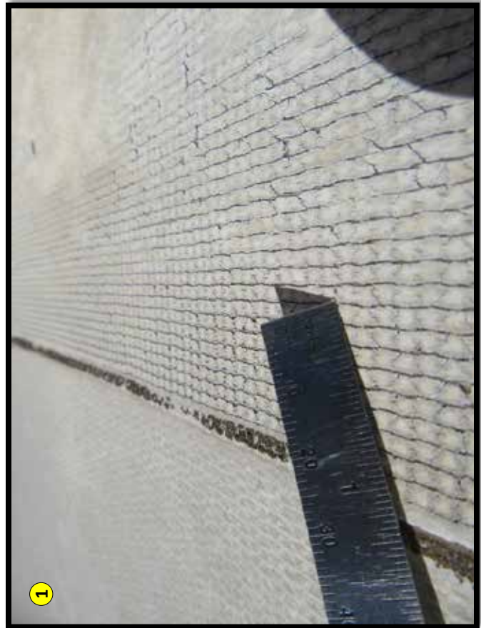
- View of Degradation to EP Roof Base Flashing
