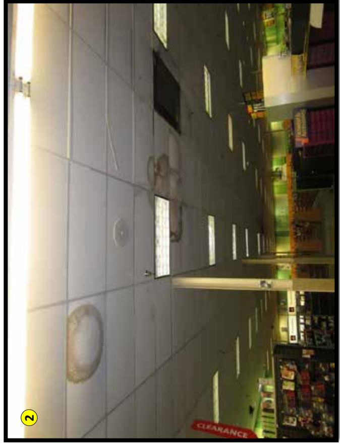
- View of Interior Retail Space Moisture Stained Ceiling Tiles
