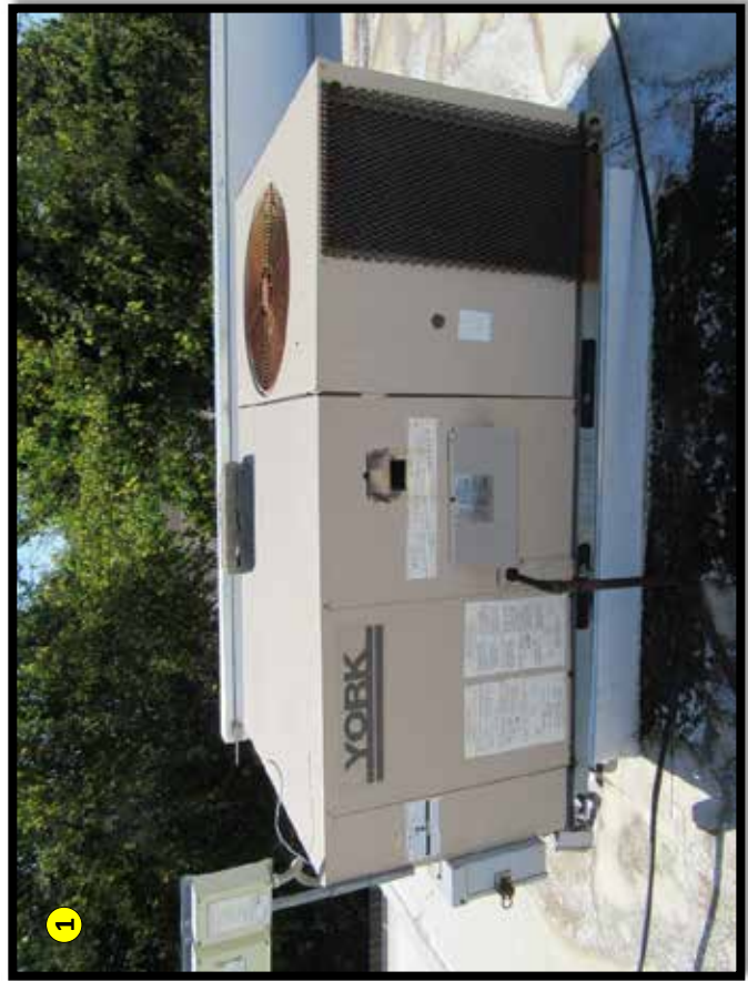
- Overview of HVAC Unit
